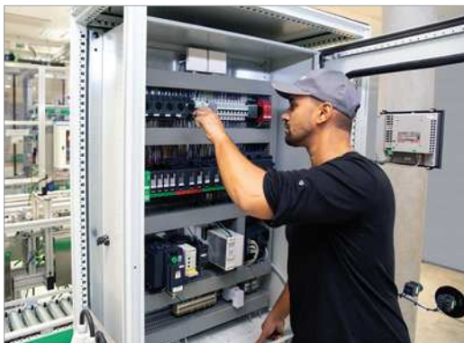
General machine control
