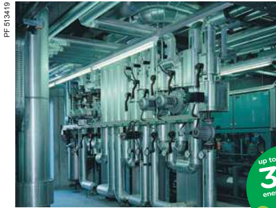
ATV12 controlling a pumping station
