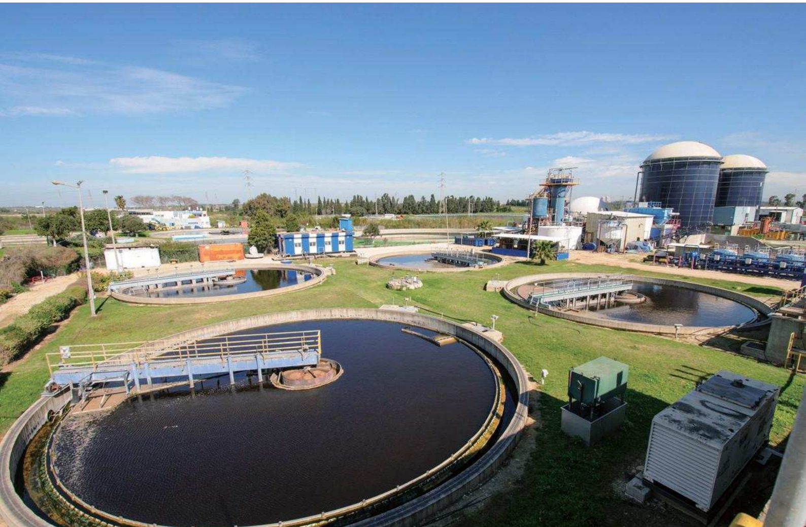
Monitoring and control at water and sewage plants
