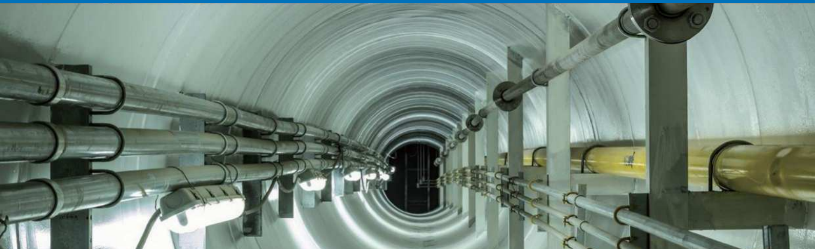
Monitoring and control of air conditioning and lighting in underground utility tunnels
